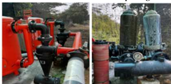
Installation of MIS Disc Filter of MIS
